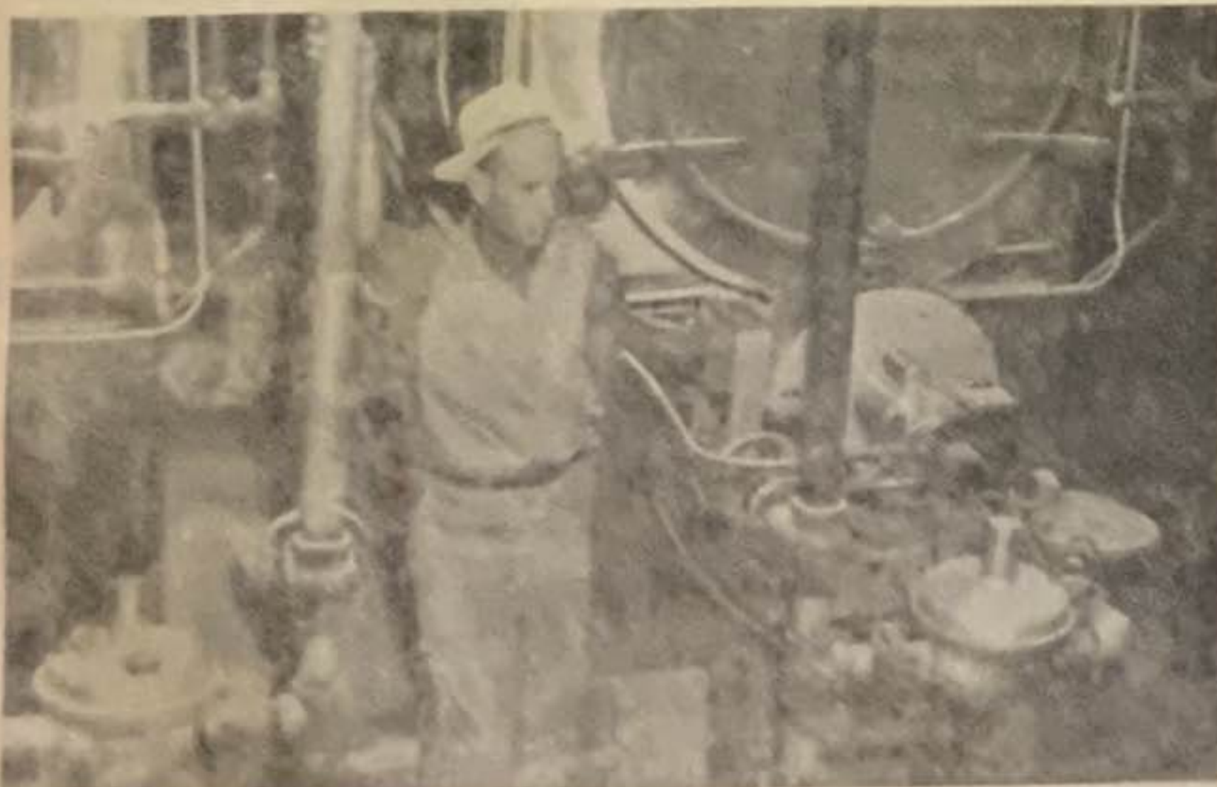
Thomas Simpson is engineer of the hospital and stands beside the two giant boilers that are the heart of the hospital's equipment. The boilers are automatically fired. The hospital also has a complete auxiliary power unit in case of power failure to the building. This is the central center of all heating, cooling and electrical wiring.
